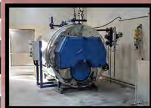
Boiler & Air Compressor Pump
