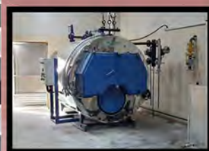
Boiler & Air Compressor Pump
